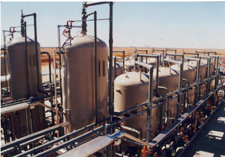
Fig.7. View of the U processing plant showing part of the IX columns for U capture.
